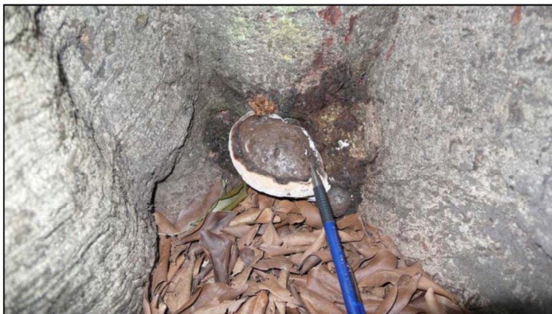
Photo H: Typical fruiting body of Phellinus sp. (Tree 1S). Ongoing rootcrown inspections and internal diagnostic testing is required to ensure the internal decay pocket does not become critical.
